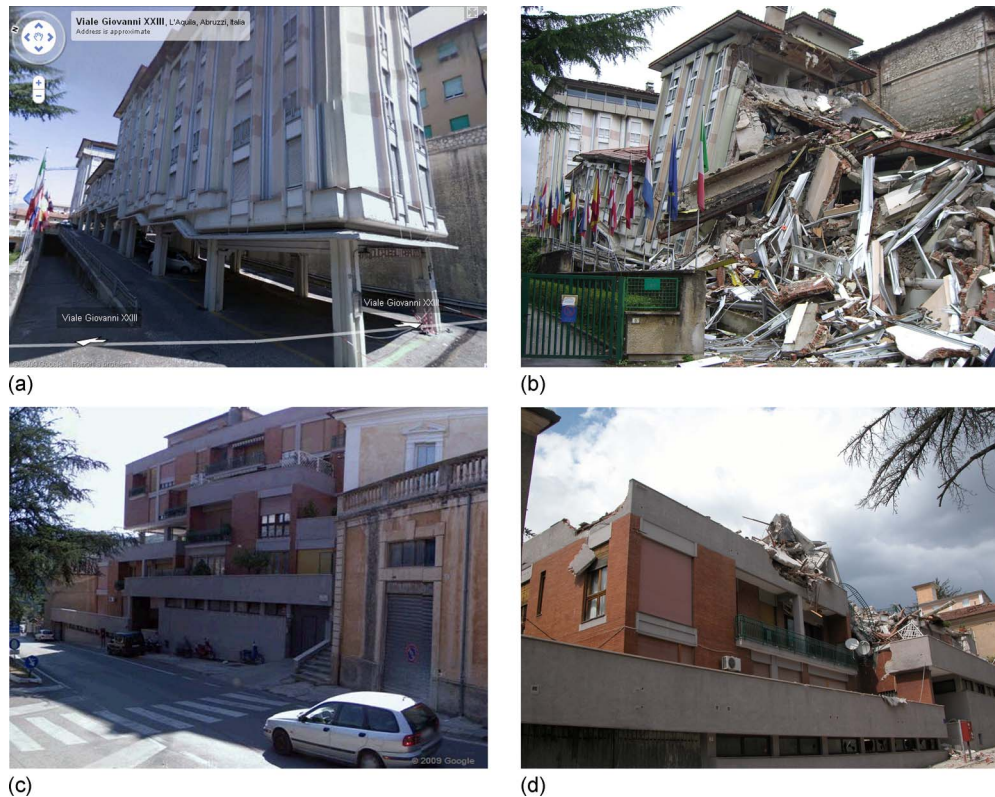
Figure 4. (a) Condition of Hotel Duca Degli Abruzzi in L'Aquila before the earthquake as obtained from Google Maps Street View and (b) the post-earthquake condition observed from the ground. It is possible to observe the presence of a significant irregularity in elevation between the ground and the first floor. (c) Before and (d) after earthquake condition of another collapsed building (irregularity in elevation at intermediate floor) in L'Aquila assessed by similar methods.
