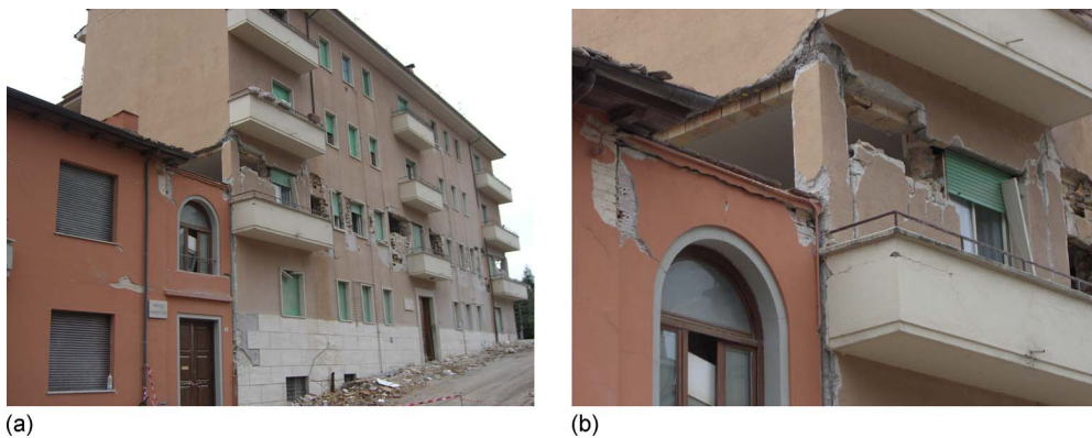
Figure 6. Perhaps unintentional vertical layout error (with the new building close to the older one with unmatched floor and roof elevations) caused pounding damage to the new building on the right.
